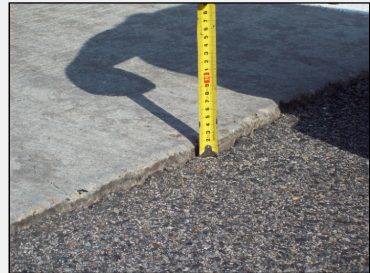
Protrusion on the boundary of asphalt pavement and concrete slab
